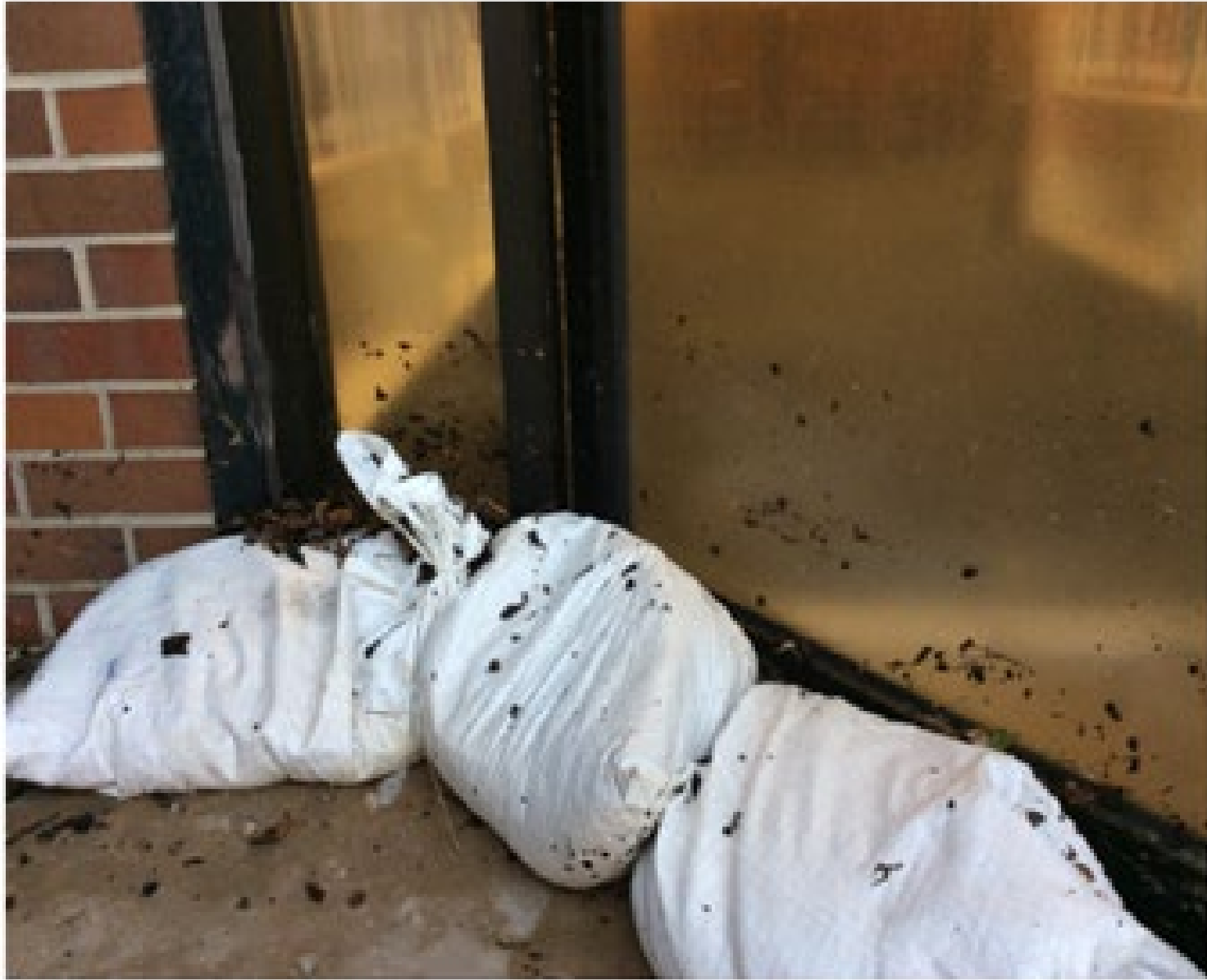
High water line evident at front entry
