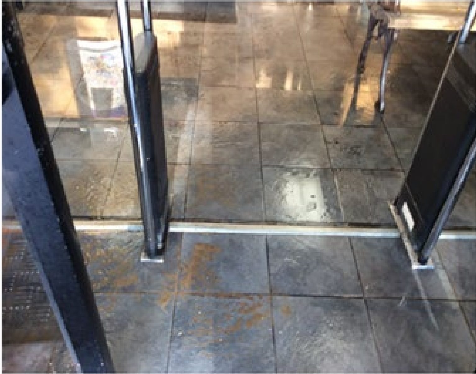
Flooding at main entry
