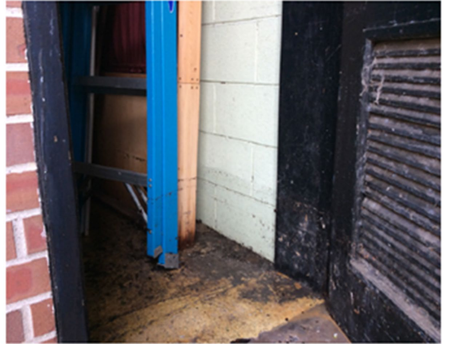
Mechanical Room high water line
