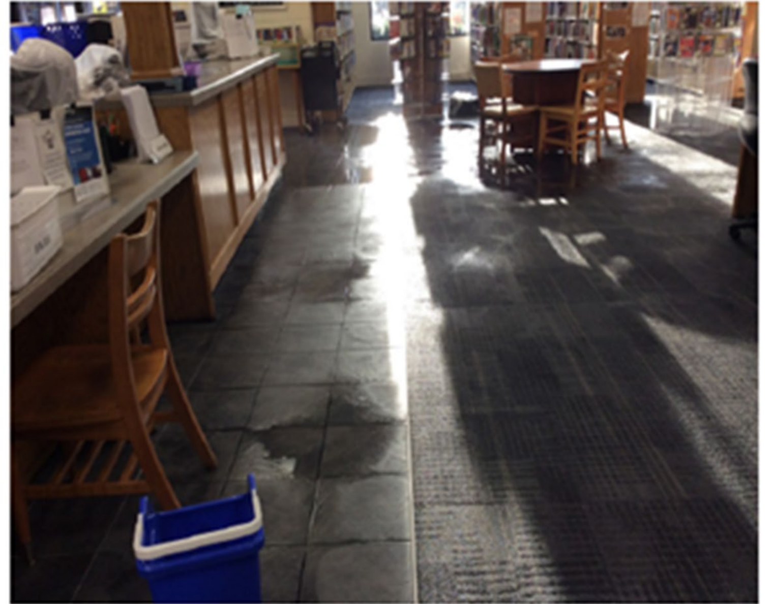
Water seen throughout library
