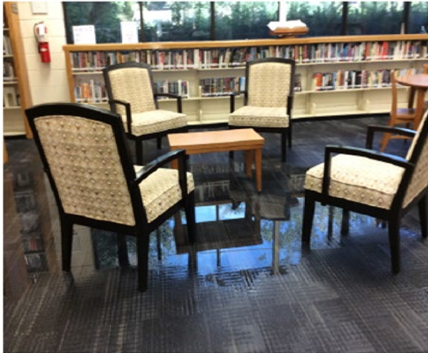
Pooling water at seating area
