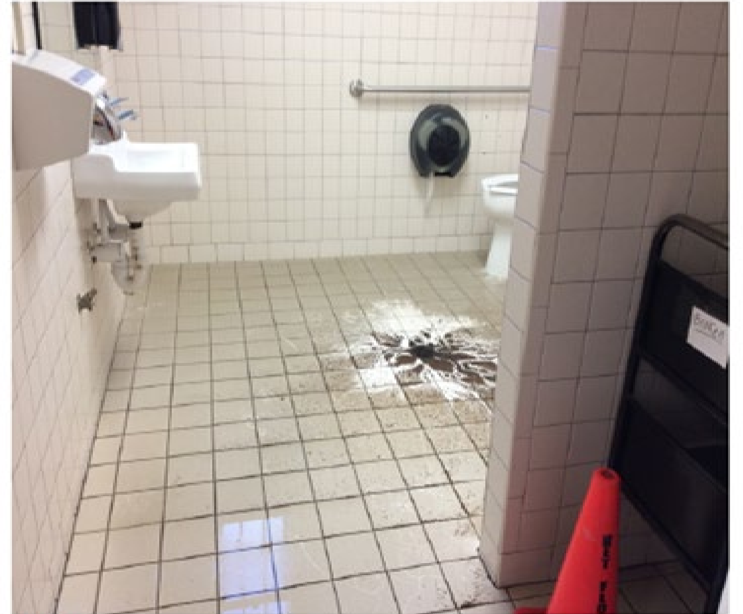
Water in restroom
